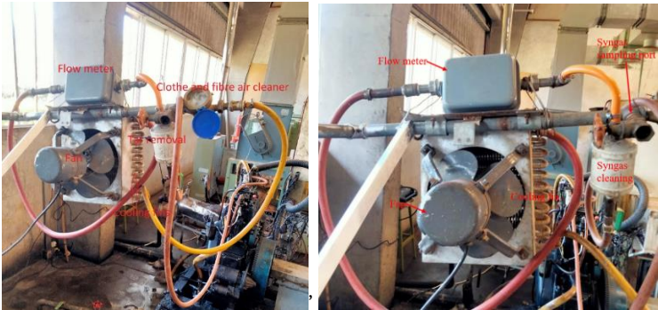
Figure 4 Syngas cleaning and cooling unit showing Syngas sampling port
