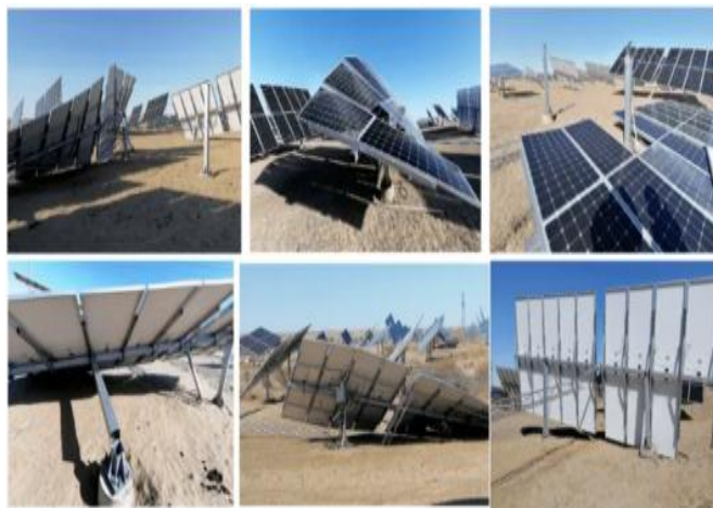
Figure 3 Accident scene of a photovoltaic power station in China due to strong winds
